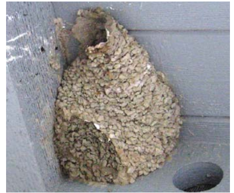
Industrious swallows at the Discovery Center have already built replacement "bottoms" for the nests that collapsed in early June.
